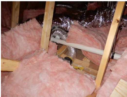
Figure 3. Disturbed attic insulation in the vicinity of a bath fan (Home A)
