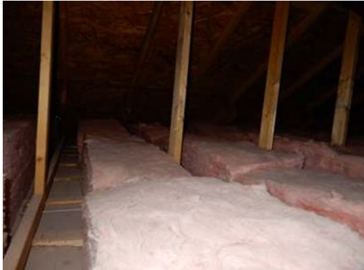
Figure 2. Large ceiling-insulation voids at Home D
