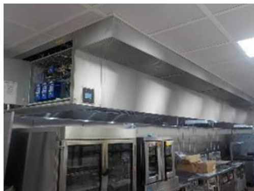
CaptiveAire hood – Main kitchen
